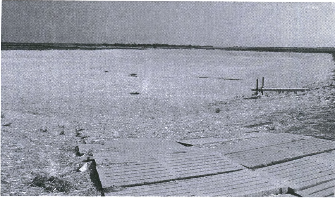
Figure 2. Permeable Straw Cover Installed on an Earthen Manure Storage Structure
